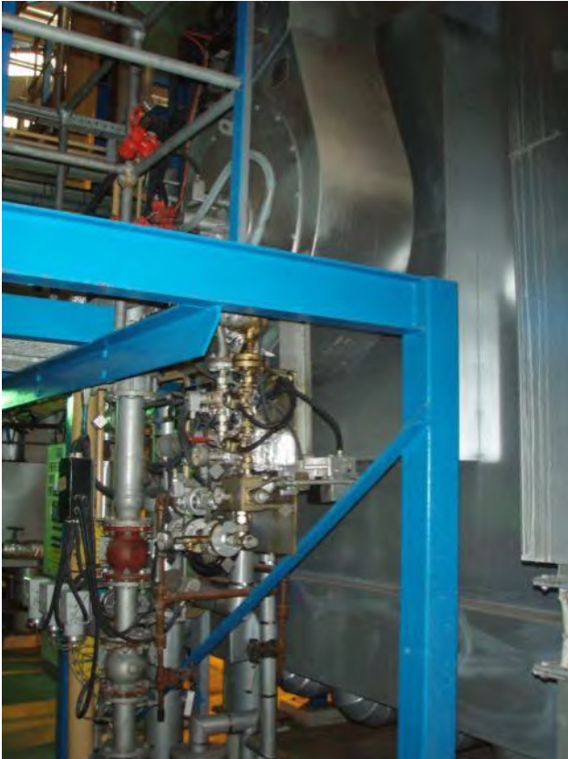
Volund Boiler Burner
